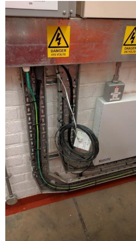
Electrical connections inside LMR
